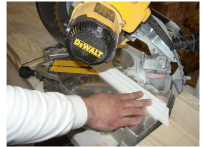
15) If base trim moldings are too long, use miter saw to cut base trim pieces to fit around bottom of column.**
