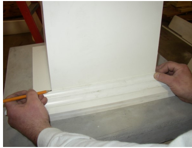
14) Use column shaft to check length of base trim molding. If trim is too long, mark cut lines for miters. Moldings should be about 1/8" longer than the width of the column.**
